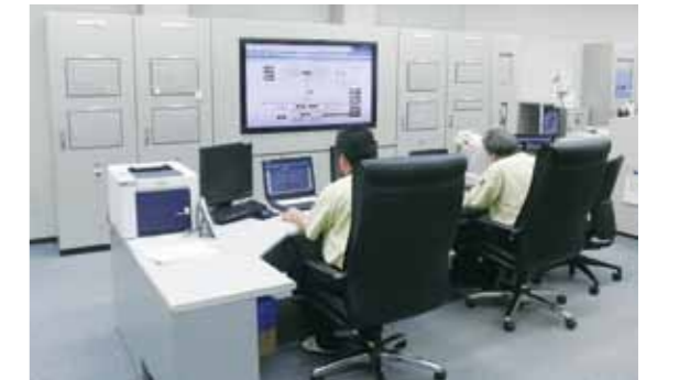
Sanrizuka Solar Power Plant
