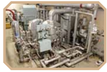
Steam turbines and generators
