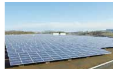
Sanrizuka Solar Power Plant
