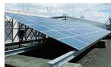
Solar panels on the NAA Head Office Building
