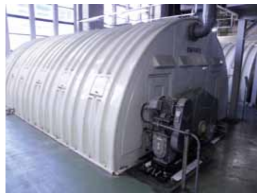
Kitchen wastewater treatment facility
