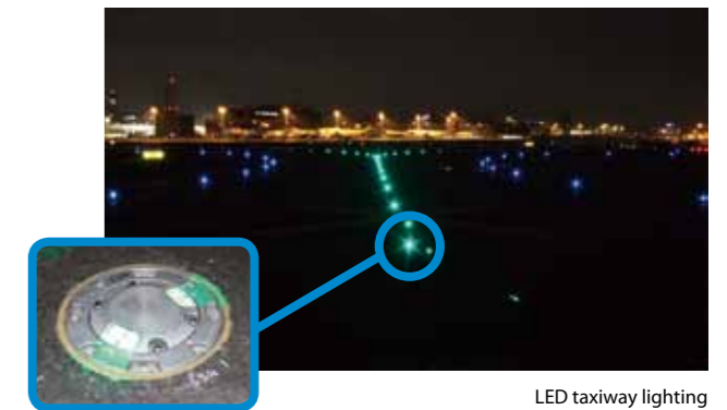
LED taxiway lighting
