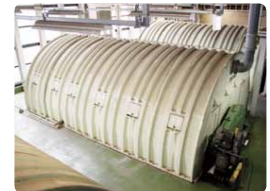
Kitchen wastewater treatment facility
